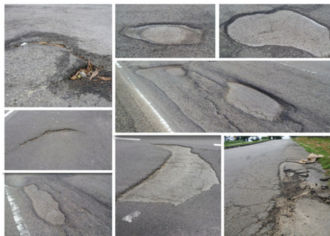
FIGURE 1. Collection of photos on pavement distresses encountered in Malaysian pavement due to poor adhesion, which includes of slippage, delamination and formation of shallow potholes
