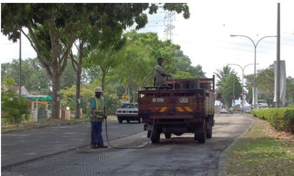
FIGURE 5. Asphalt emulsion tack coat application using hand wand sprayer in Malaysian road construction
