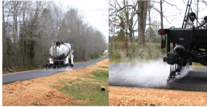
FIGURE 4. A view of asphalt distributor truck performing the tack coat application on a road section to be paved (West et al. 2005)
