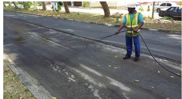
FIGURE 7. Typical poor construction quality due to insufficient knowledge related to pavement bonding. Pavement surface remains wet after milling operation during the tack coat application. Clearly visible also the existence of organic matters (leaves) which can hinders the bond development between pavement layers
