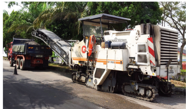
FIGURE 2. Wirtgen milling machine W1900 used by the contractors to perform milling operation
