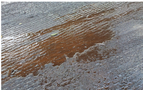
FIGURE 6. Ponding of asphalt emulsion tack coat at certain location on a pavement. Excessive application of the tack coat initiates the slipping plane for which distresses like delamination and slippage failure to occur
